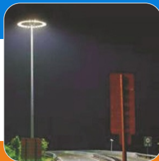
Street High Mast Pole
